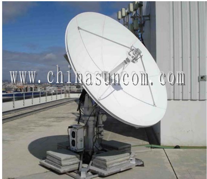
2.4m antenna installed in Portugal
