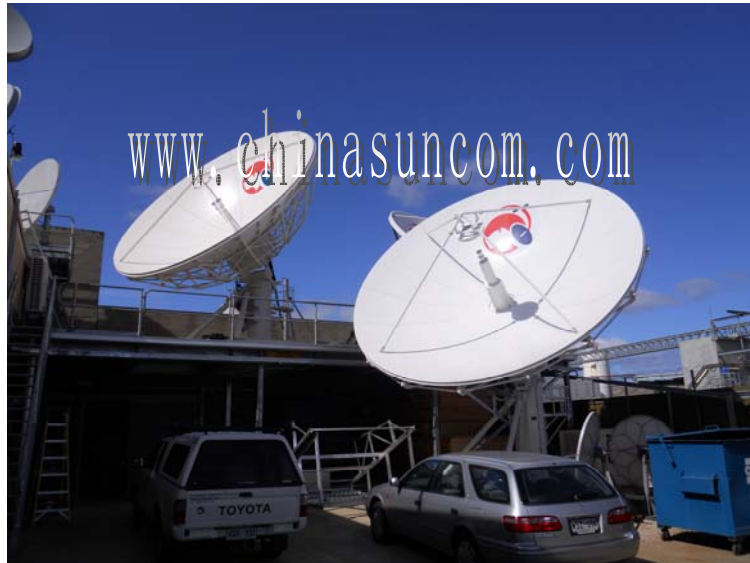
6.2m antenna installed in Australia
